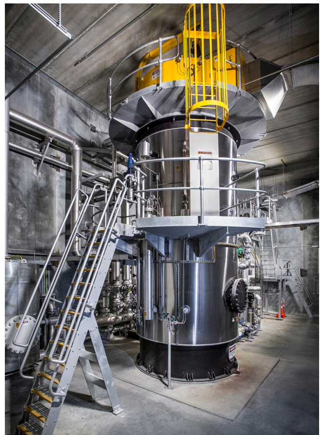
Electrode Boiler operating at Synlait Dunsandel.
